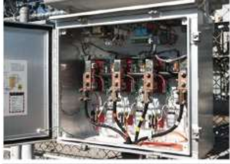
Figure4: PLC Substation Equipment
