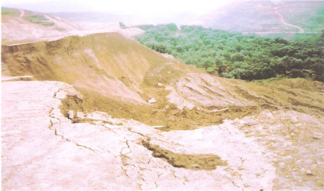
Figure (2): Failure of a 16 m high highway embankment founded on a thick layer of colluvial deposits along Amman-Jerash highway at St. 38+600
