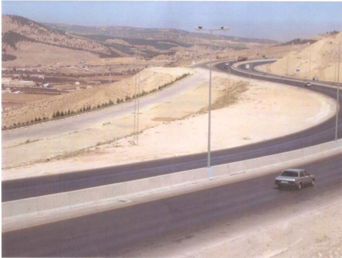
Figure (13): Shifting of a section of Jordan Road due to a continuous creep movement of the road embankment constructed in an area that suffered from an old landslide
