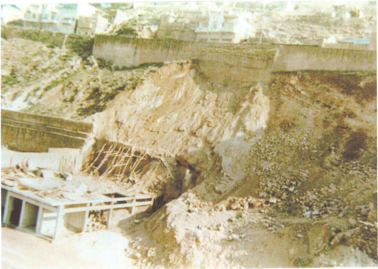
Figure (11): The construction activities at the toe of Jebel Jofeh that led to slope failure and closure of the upper road
