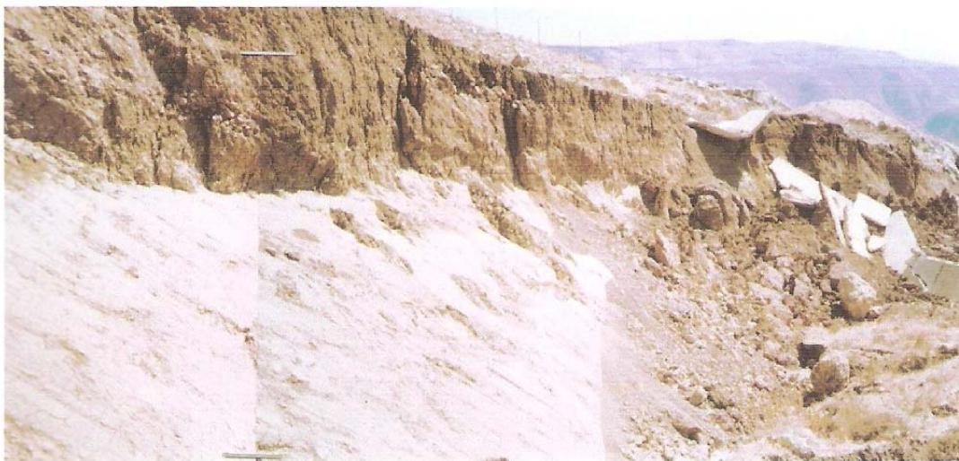
Figure (3): The sliding surface at the top of clayey marl bed in Wadi Es-Sir Sewage Treatment Plant. Note the jointed cliff of the limestone overlying the marl that belongs to Naur Formation (A1/2)
