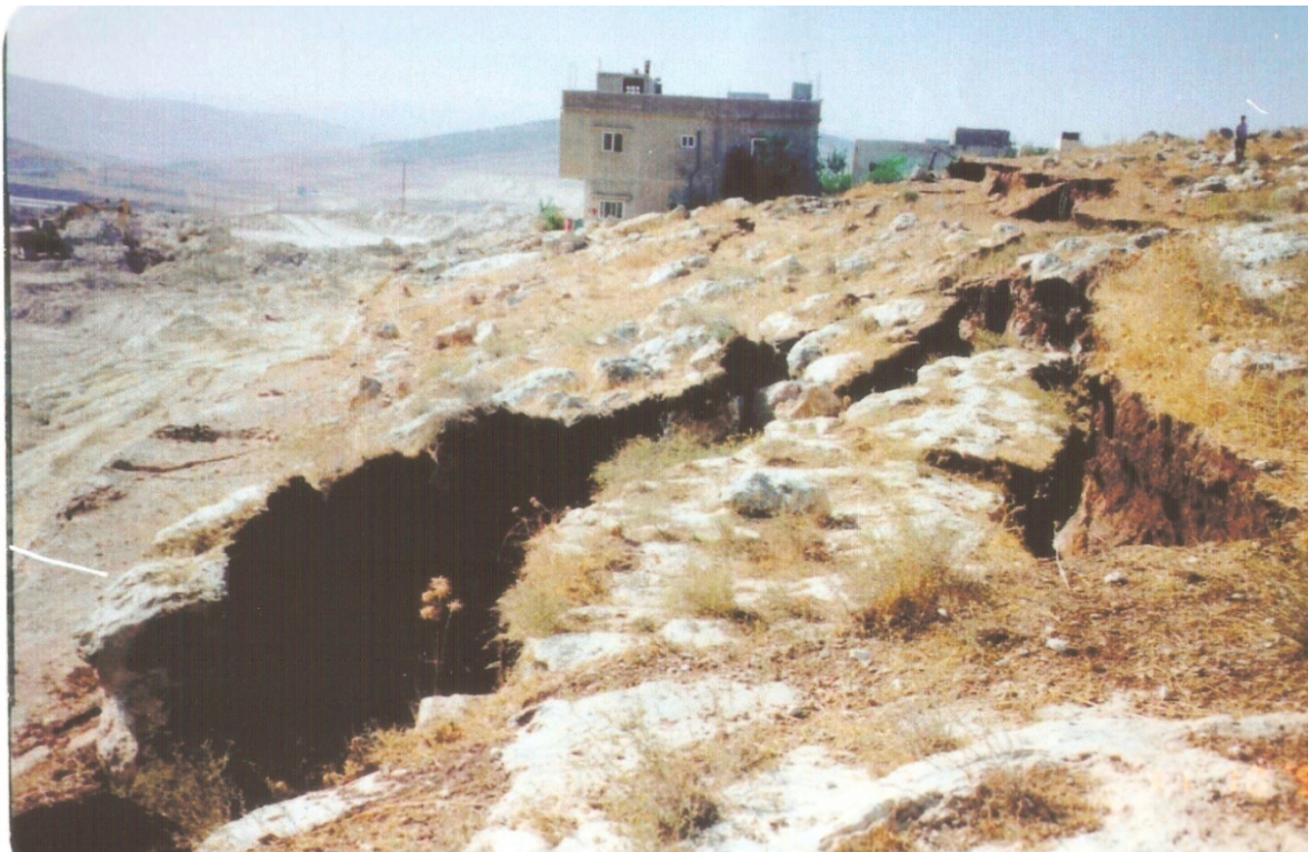
Figure (12): Failure along Amman-Jerash-Irbid highway due to the daylighting of the wet plastic clayey marl that resulted in the collapse of the houses near the edge of the excavation
