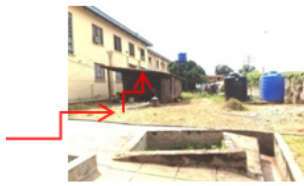
Figure 22: North View; erosion along the Path to Open Sun Drying Hangers
