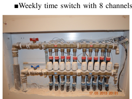
Fig. 7: Under Floor heating (UFH) Cabinet [theben values] M.K villa
