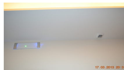
Fig. 9: Motion detector Ground Floor.(passage). in M.K villa
