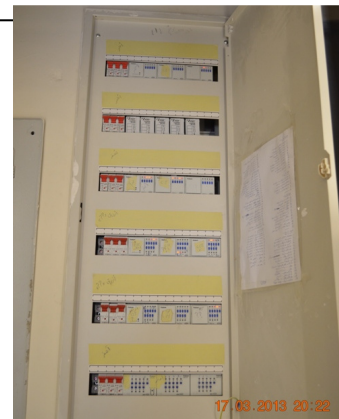
Fig. 6: HACP / Home Automation control panel in Ground floor M.K villa
