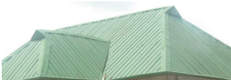
Plate 2: Aluminium used for Roofing Source: Author's fieldwork.2011
