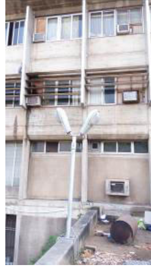
Plate 6: Units mounted on windows and walls in a haphazard fashion (Source: Author, 2016)
