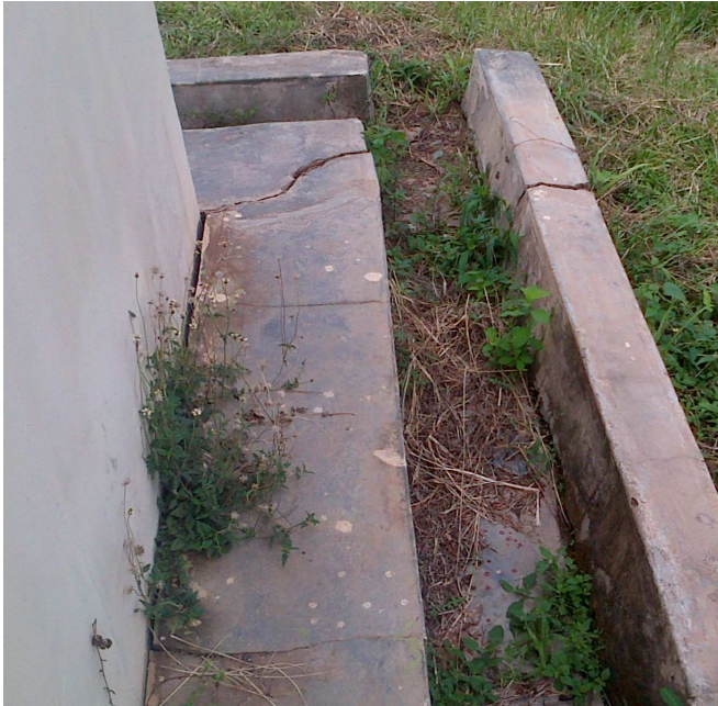
Figure 2: Distressed Building in the Study area Showing Cracks on the wall of BACOSA Extension I
