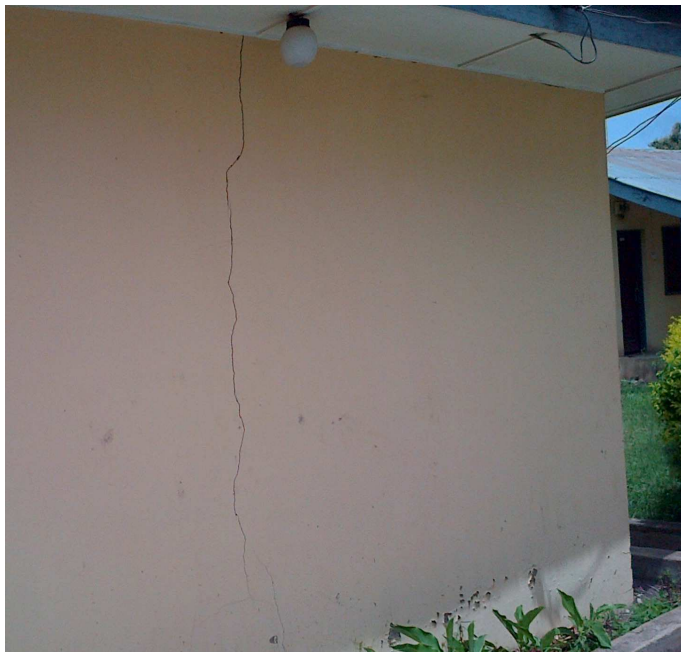
Figure 4: Distressed Building in the Study area Showing Cracks on the wall of BACOSA Extension II
