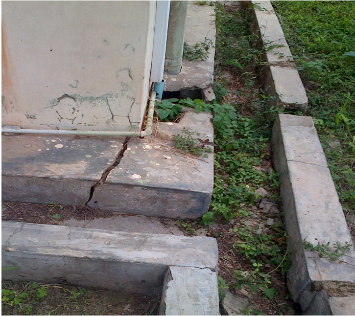
Figure 1: Distressed Building in the Study area Showing Cracks on the wall of BACOSA building
