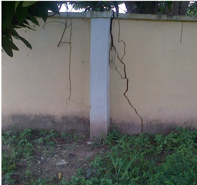
Figure 3: Distressed Building in the Study area Showing Cracks on the wall of a fence behind BACOSA Extension I
