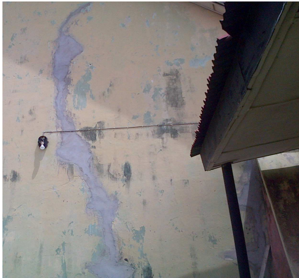
Figure 7: Distressed Building in the Study area Showing Cracks on the wall of 200Level Physics Lab.
