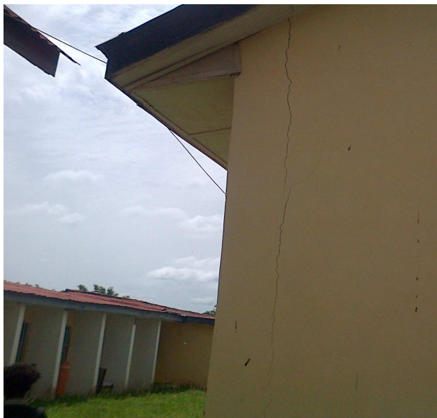
Figure 8: Distressed Building in the Study area Showing Cracks on the wall of Faculty of Science building
