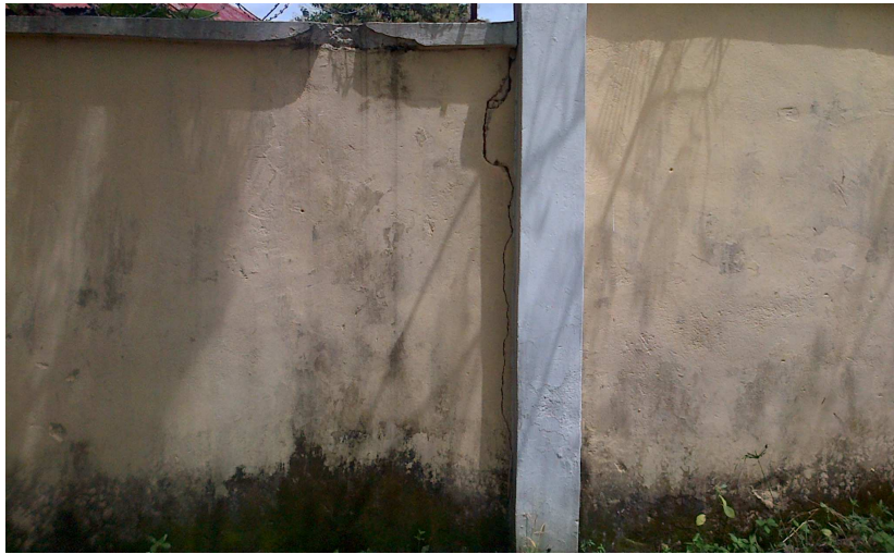
Figure 5: Distressed Building in the Study area Showing Cracks on the wall of fence behind MICOM Lab.
