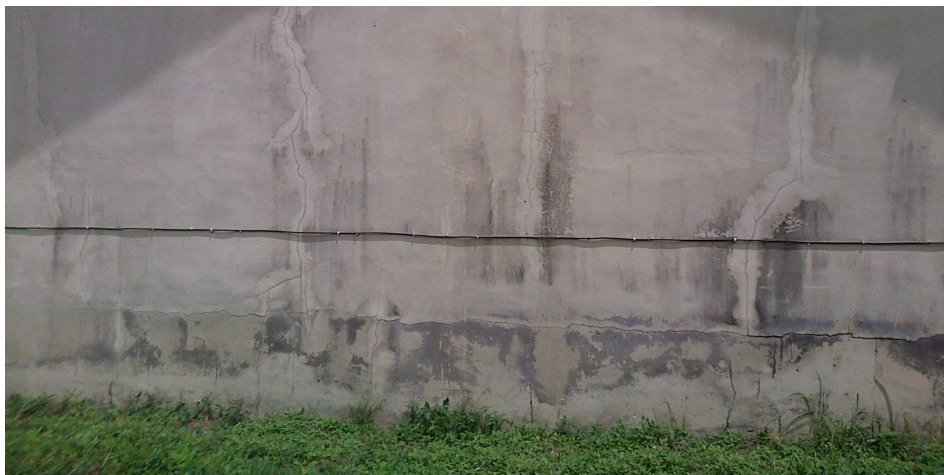
Figure 6: Distressed Building in the Study area Showing Cracks on the wall of General Lab
