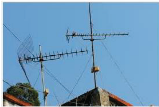
Figure 4: Yagi-Uda antenna placed on the roof.
