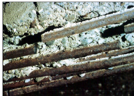
Fig. 1. Beam: corrosion destruction of concrete cover; fragile fractures of the longitudinal and transversal steel reinforcements by stress corrosion cracking.
