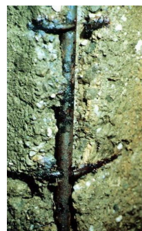
Fig. 3. Column: corrosion of concrete cover; fragile fractures of the steel stirrups by stress corrosion cracking.
