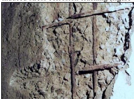
Fig. 4. Wall: local spalling of concrete cover; fragile fractures of the steel reinforcements by stress corrosion cracking.
