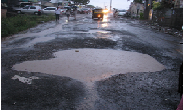
Figure 3: Formation of potholes on road due to poor drainage of road surface
