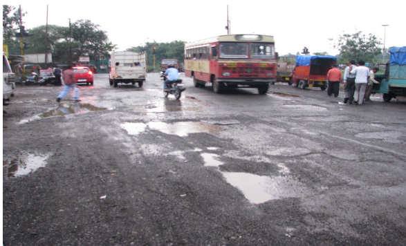
Figure 2: Accumulation of Aggregates on Road Sides
