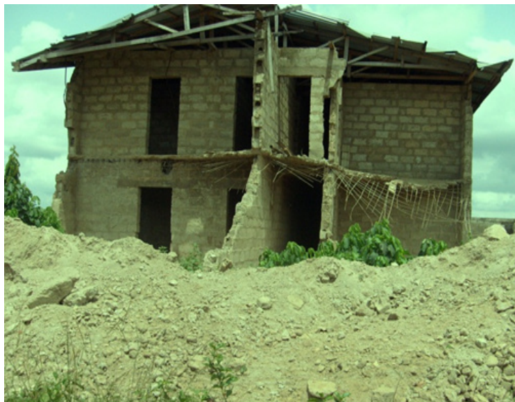
Plate 1: A collapsed one-story building
