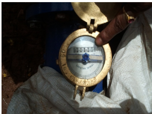
Figure 2. Bulk Flow Meter at Lingarajnagar, Hubli
