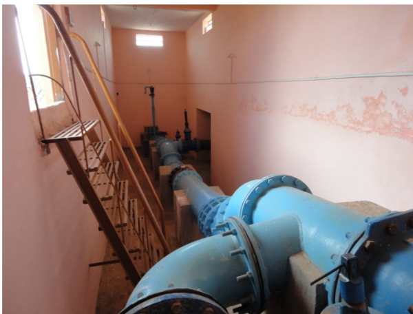
Figure 4. Bulk water Meter and Valve Control Room near Nrupathunga Betta Tank, Hubli
