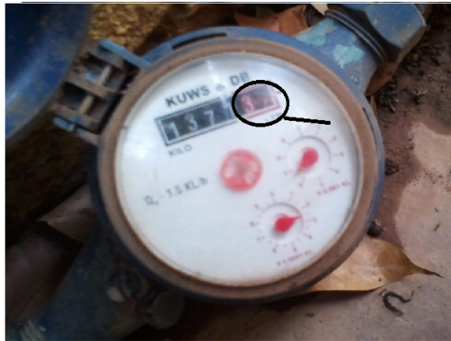
Figure 3. Customer Meters at Lingarajnagar, Hubli
