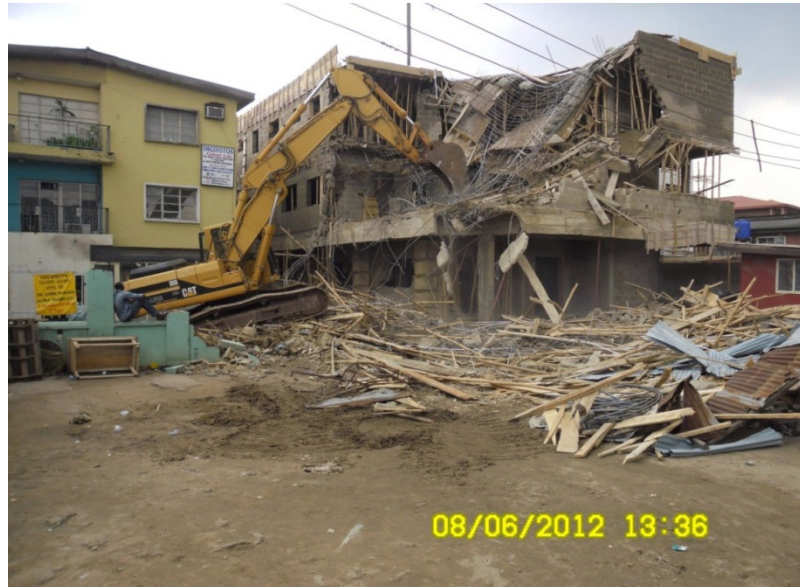
Figure 4: Collapse site at 13 Awolowo way Ikeja Lagos State, Nigeria
