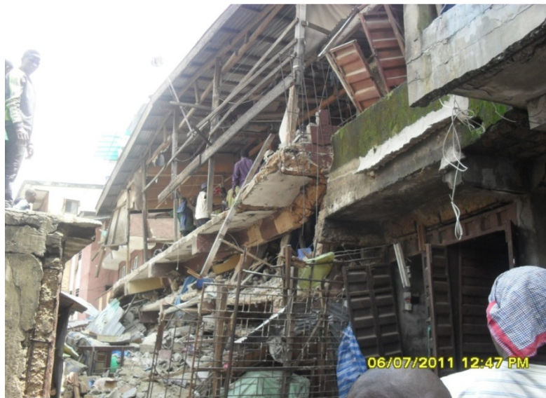
Figure 5: Collapse site at Idunmota Lagos State, Nigeria
