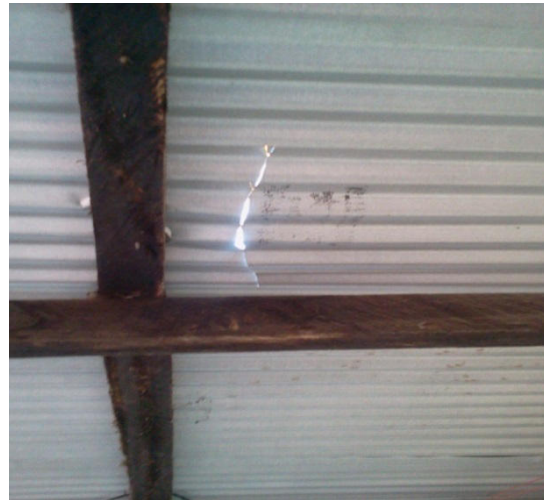
Plate 7: Damaged roof from flying rocks
