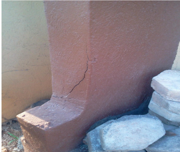
Plate 6: Cracked Walls due to vibration
