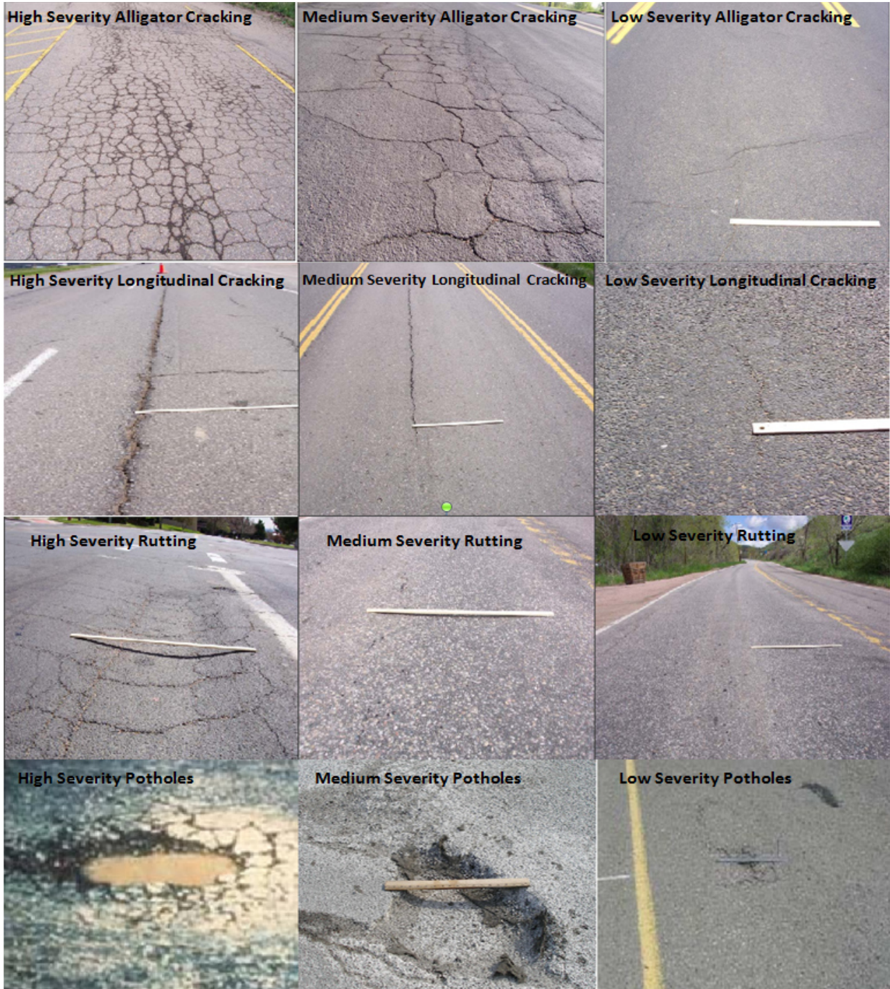
Plate (1): Selected photographs of main kinds of surface pavement distresses
