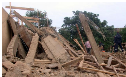
Figure 2: Collapse of a Hospital Reconstruction in Benin City Source: http://news.naij.com/812.html
