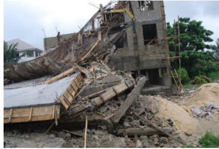
Figure 3: Collapse of Two storeys Building in Port Harcourt
