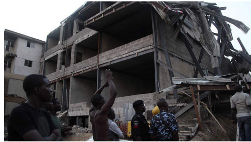
Figure 10: Collapse of Twin four Storey Building in Lagos
