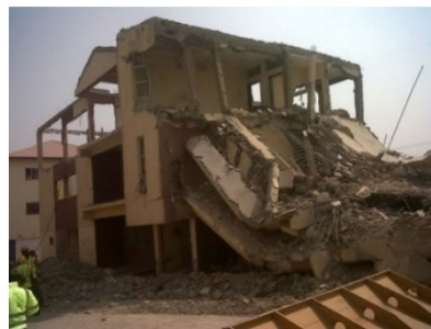
Figure 8: Collapse of Three Storey Building in Abuja
