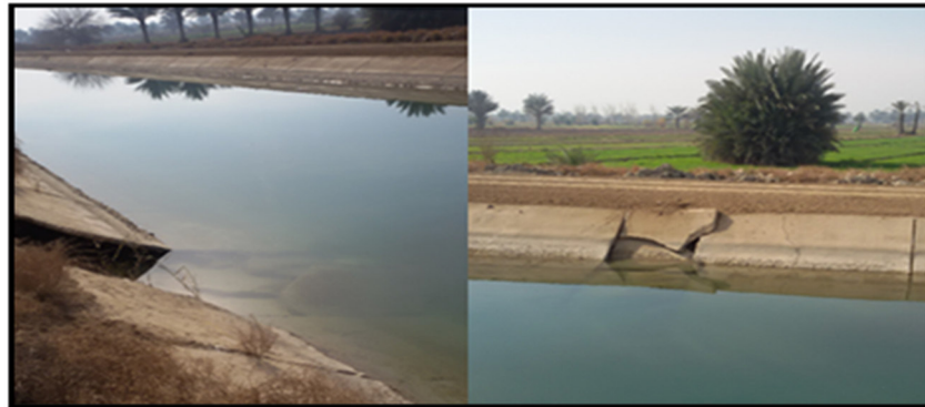
Photo (1) collapses and cracks in the layers of lining of Hilla main canal
