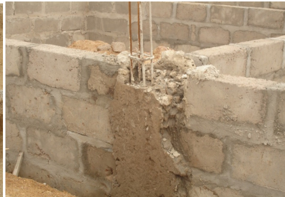
Plate 2: A Bulged Column due to Poor Quality Formwork used
