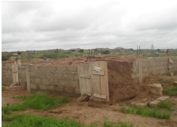
Plate 7: Evidence of the Result of using wrong Consolidation Equipment for Hardcore Filling
