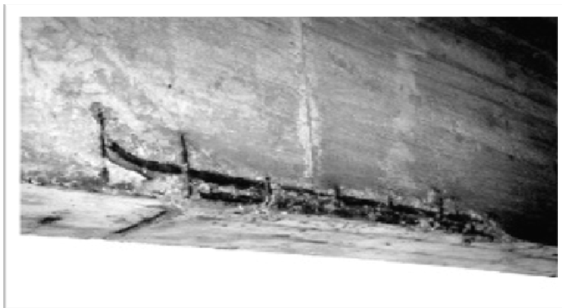
Figure 4: Concrete spalling in a low cover zone (Costa and Appleton; 2002).
