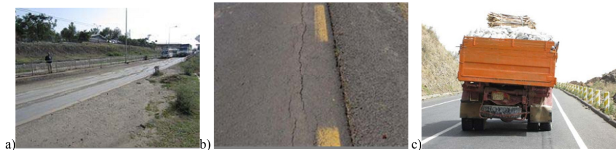
Figure 2 (a) Urban trunk road under the influence of black cotton soil, Rutting occurred on the surface. (b) Rural trunk road - Vertical rutting of pavement edge. (c) Heavy vehicles hauling lime-stone have been passing in Abay. Travelling speed is lower than walking speed. [15]
