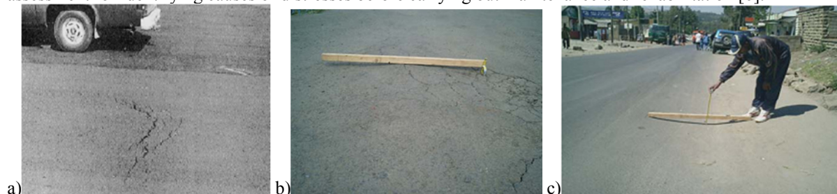
Figure 1(a) Slippage cracks, (b) Swelling- upward displacement of a pavement, c) Sag in asphalt pavement [12]
