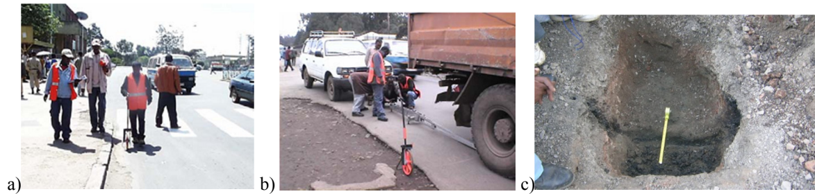
Figure 3 (a) and (b) Visual Condition Surveys [12]; (c) Test pit on Addis - Jimma Road [5]
