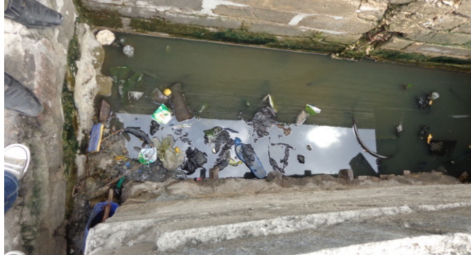
Figure 7: Blockage of natural water flow
