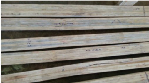
Plate 6: Bending failure in glulam
