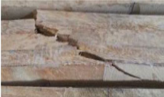
Plate 2: Bending failure in glulam
