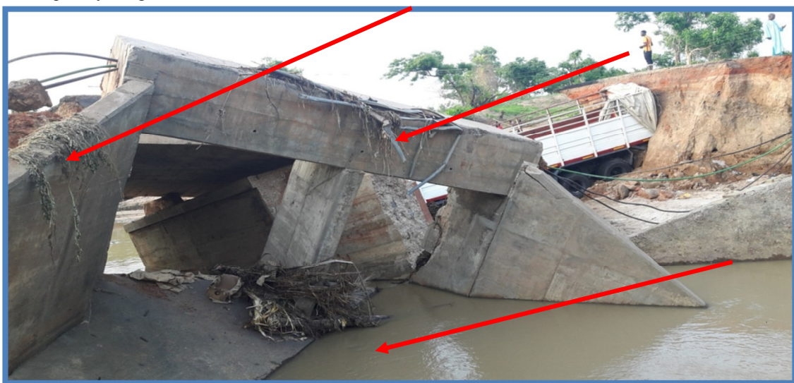
Plate 1: Image showing remnant debris
