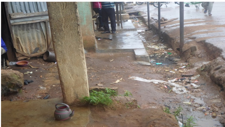
Plate 2: Blocked drainage from informal sector activity
