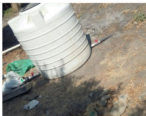
Figure 2: The settling tank
