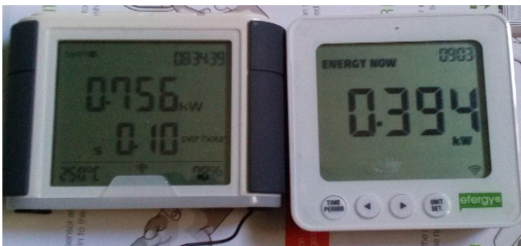
Fig 4: Wireless Energy Monitoring Devices Indicating Readings.
