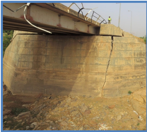
Figure 26. Major cracks on abutment.
