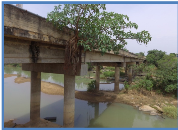
Figure 14. Tree growing on bridge fascia. Source: Field Survey 2019
