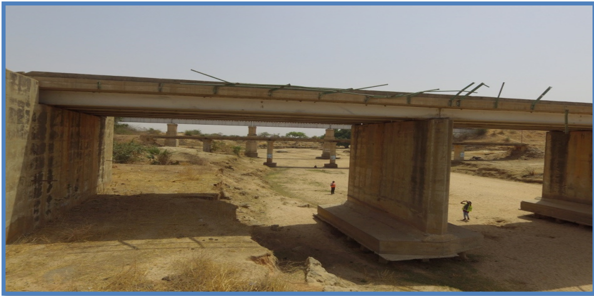
Figure 24. Major loss of channel bed to erosion and scouring. Source: Field Survey 2019
