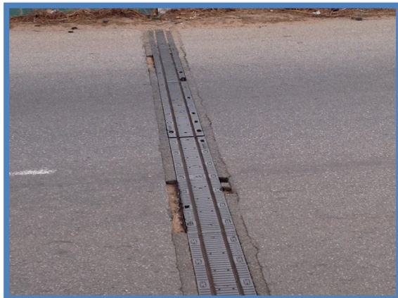
Figure 3a. Deteriorating expansion joint
