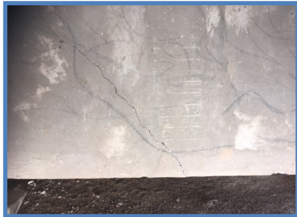
Figure 18. 3mm wide crack on approach beam
