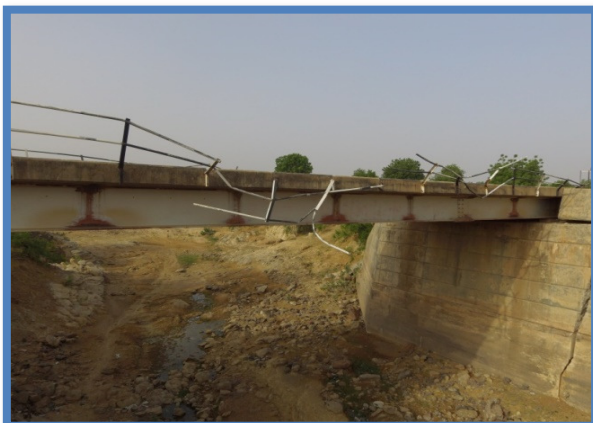
Figure 28. Poor attempt to arrest backfill loss. Source: Field Survey 2019
