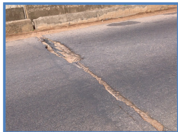
Figure 3b. Deteriorating expansion joint.
