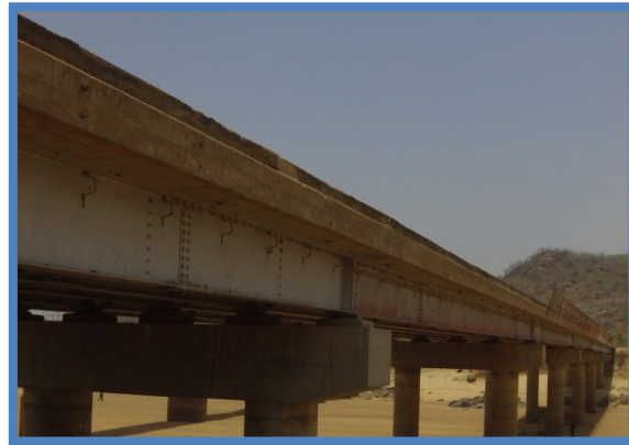
Figure 20. Missing railings due to vandalism.
