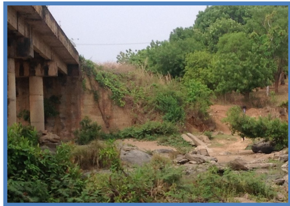
Figure 10. Unwanted vegetation on embankment.
