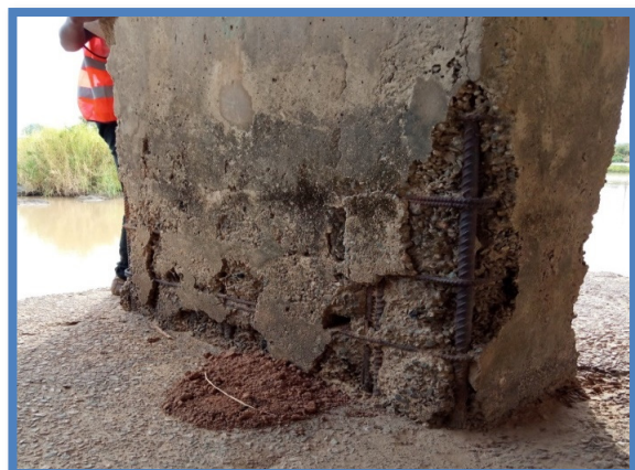
Figure 5. Exposed rebar with section loss
