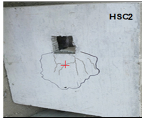
Plate (8) Tension Face for Slab HSC2
