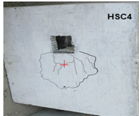
Plate (10) Tension Face for Slab HSC4
