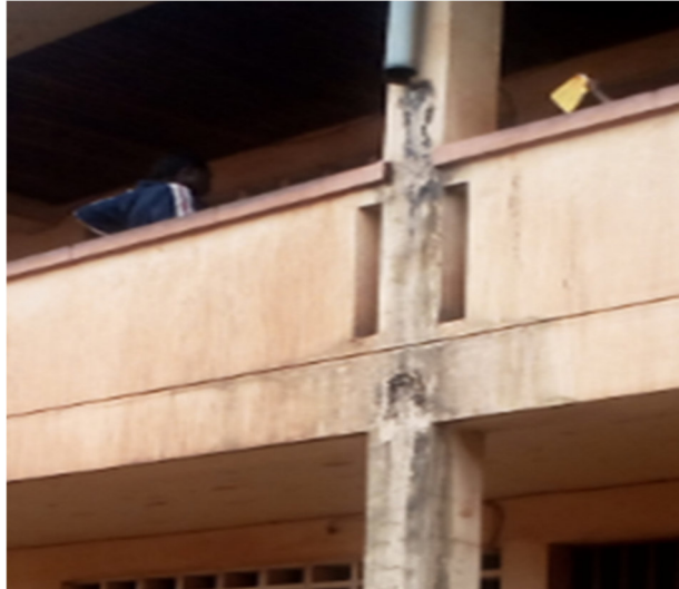
Figure 9. Defective water descent
