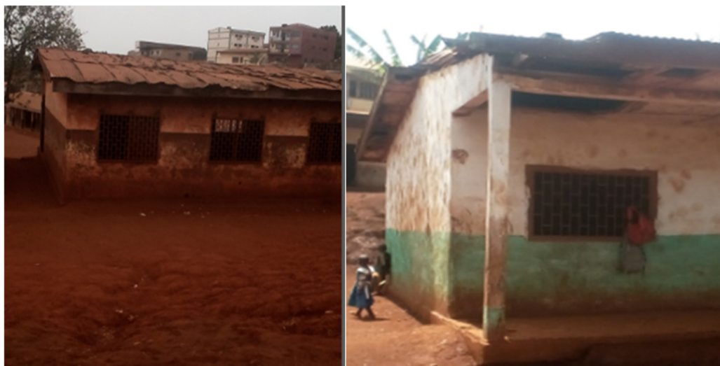
Figure 16. Poor paint condition / paint aging
