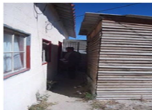
Figure 5.6 An informal extension on the backside of a row house. The entrance is blocked by the informal structure creating difficult access and limiting air circulation, a reason for guided densification.
