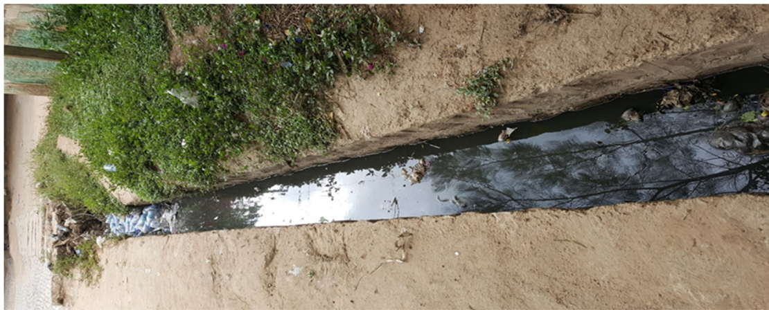
Figure 4: Solid waste and dust accumulation in the drainage system and creates water stagnation in the side channel
