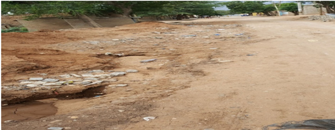
Figure 6: Eroded roads and gully formations due to lack of side ditches
