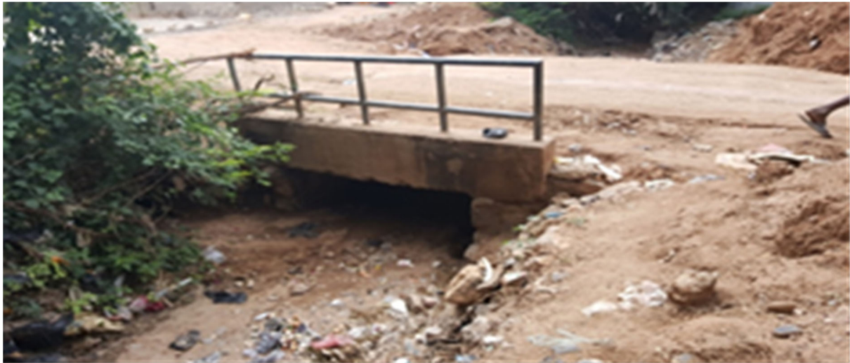
Figure 3: Almost all filled with the sedimentation of side ditches
