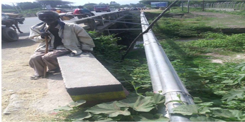
Figure 6: Cross section of Bishan Guracha Water Supply Pipe on Tikur Wuha River
