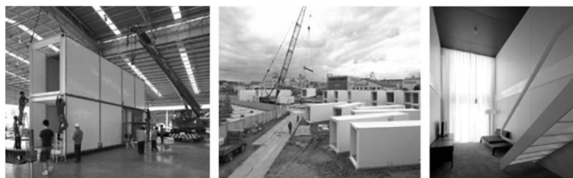
Figure 5. (Left) Full container assembly in factories after 2011 Japan earthquake and tsunami. (Middle) Container deployment at sites (Right) The container is interior. Source: (Hany Abulnour, 2014).
