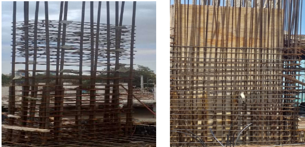
Fig. 4.5. Improper lapping zones observed during site over survey
