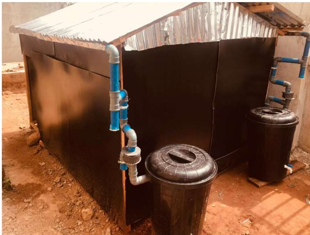
Plate 1: The Prototype RWH system components
