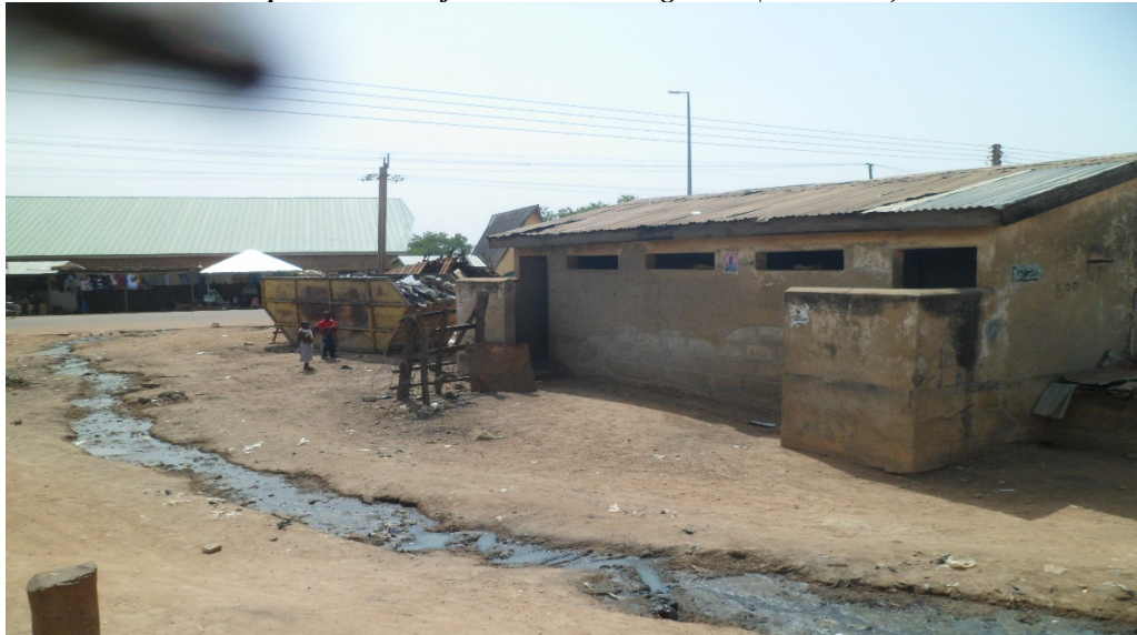
Plate 4.0. Shows the deplorable state of MAPT at the Zongo area (KVIP toilet)
