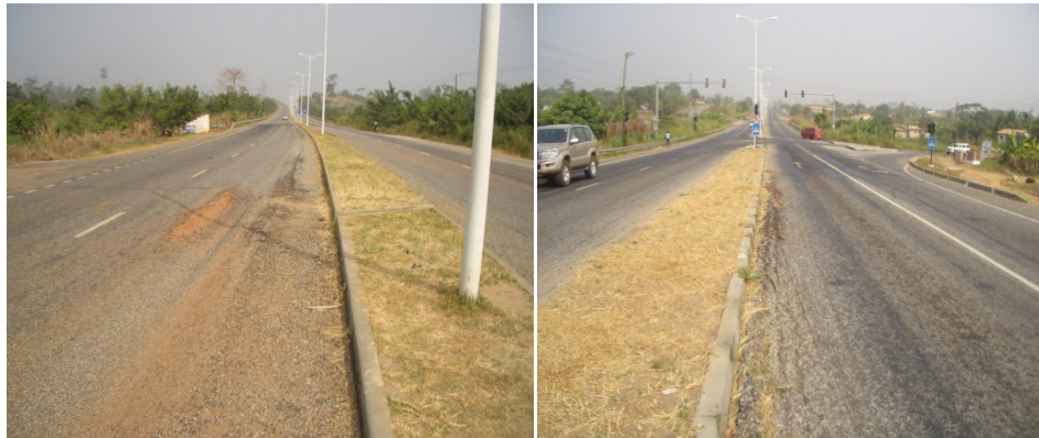
Road defect (pothole) Shoving and Longitudinal grooves
