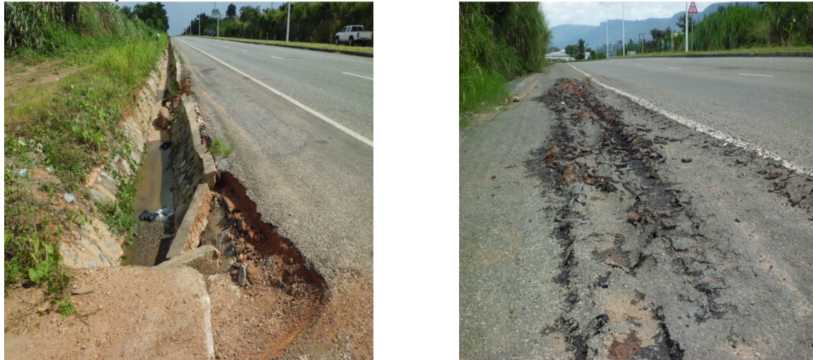
Fig 1: A 3- month old road surface showing poor drainage works and premature road surface failure.
