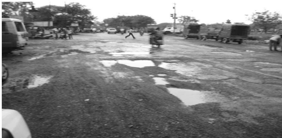
Figure 7: Formation of potholes due to Poor Drainage
