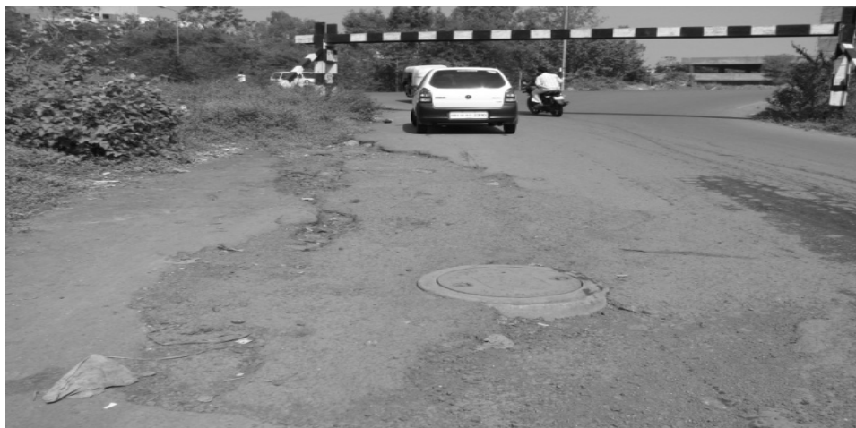
Figure 11: Cuts in roads due to the flow of water
