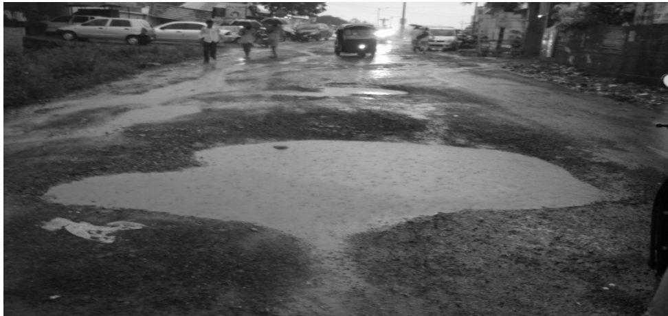
Figure 9: Formation of potholes due settlement of sub grade
