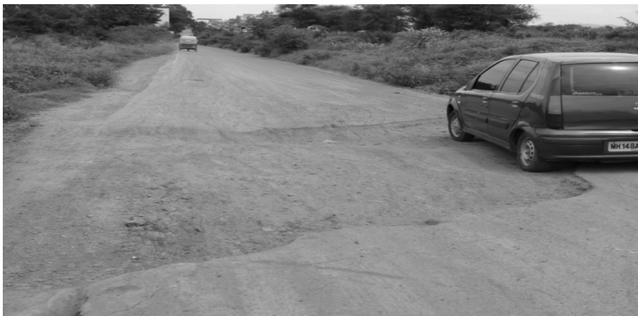
Figure 2: Cuts in road due to water
