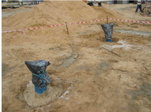
Plate 3: Another two Wells drilled for the purpose of groundwater control at site
