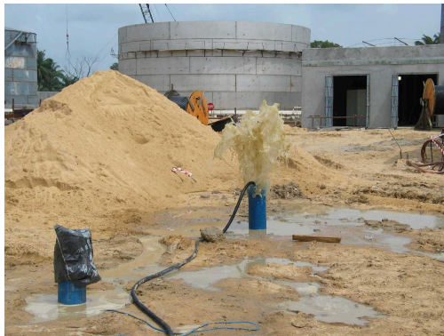
Plate 2: Two of the Well used in Pumping test analysis
