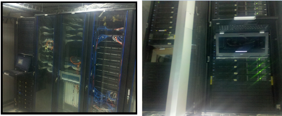
Figure 3.1: Swift Network Three-Tier DCN (Source: No 3 Isaka Tinubu, Victoria Island Lagos, 2012).
