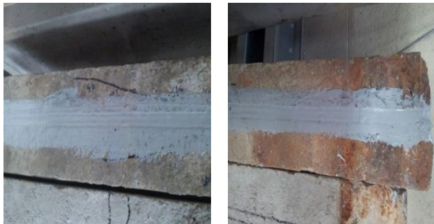
a. A1T Control.Beam b. A1CL3 Corroded. Beam
