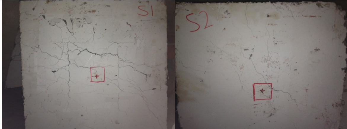
Figure (2) Failure Mode of Panel (S1)
