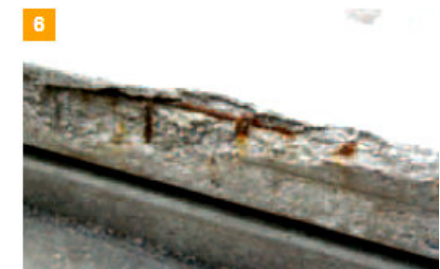
6 The viewer sees the corrosion damages like that.
