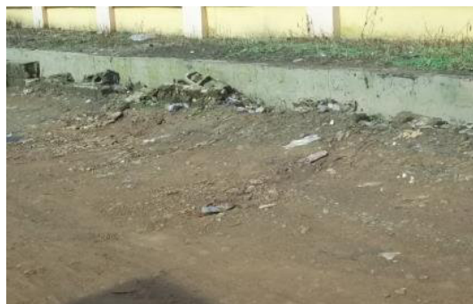
Plate 7: A Badly damaged Drain at Dele Johnson Street Due to Improper Construction
