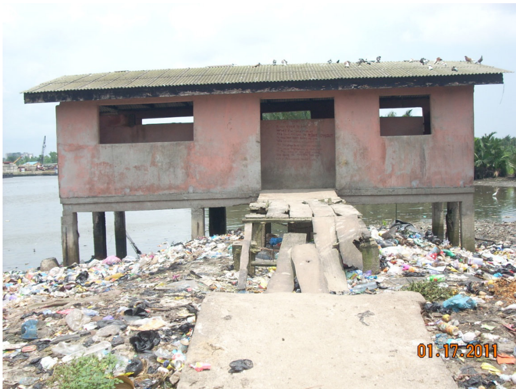
Plate 2. Garbage Dump Close to Pier Toilet, Amadi-Ama (Source: Authors' Field Survey, 2011)
