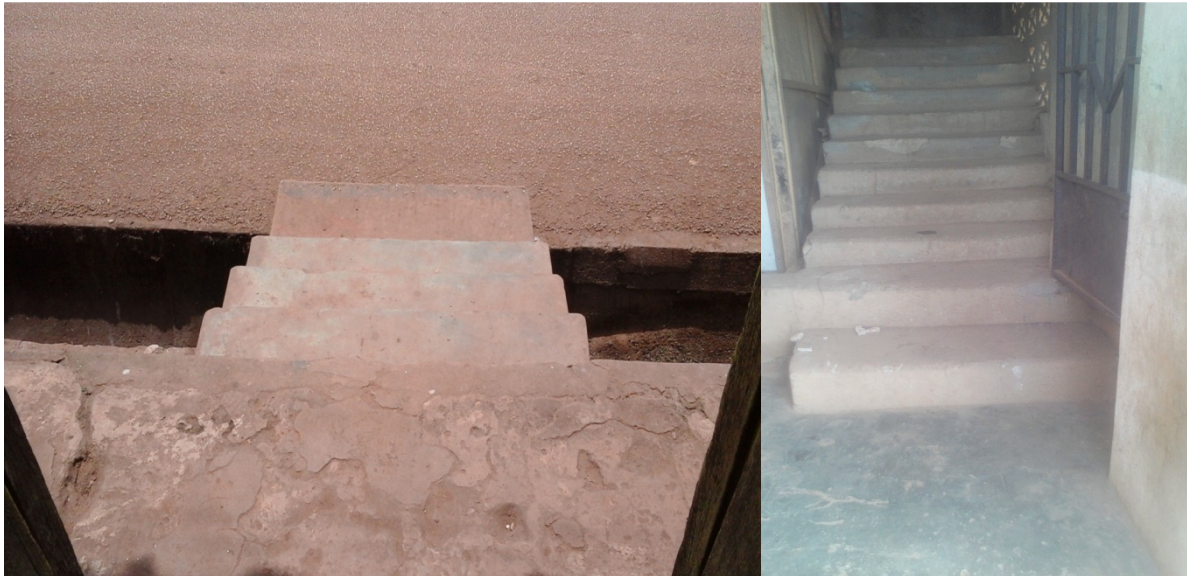
Figure 2. A stair in one of the compound houses in the selected neighbourhoods Source: Field Survey (2015)
