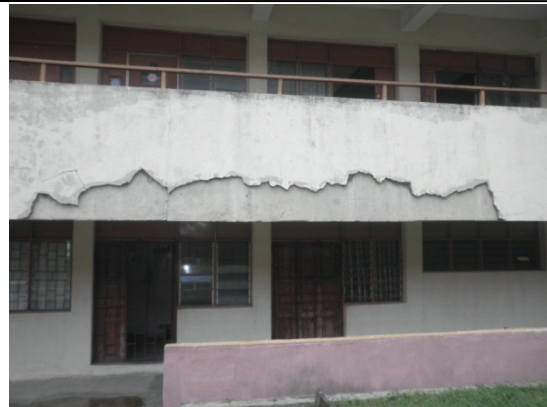
Plate 4: Ripped off concrete Plastering (Author's survey 2012)
