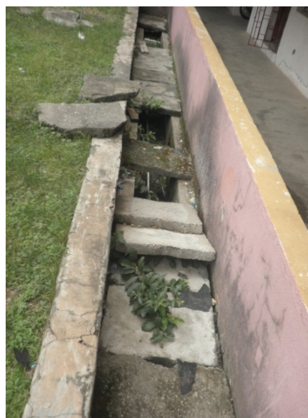
Plate 2: Drainage over-grown with weeds (Author’s survey 2012)
