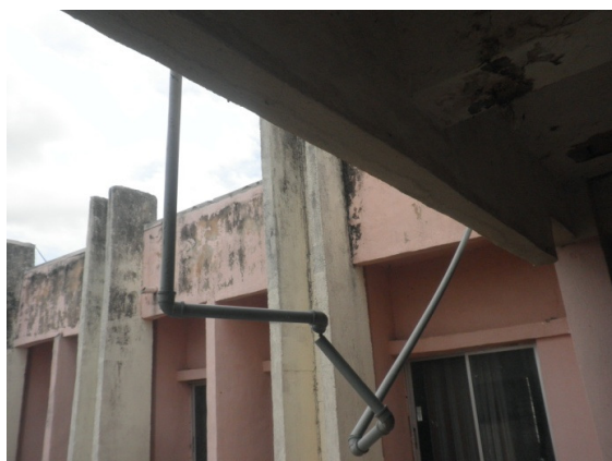
Plate 7: Damaged water pipes (Author's survey 2012)
