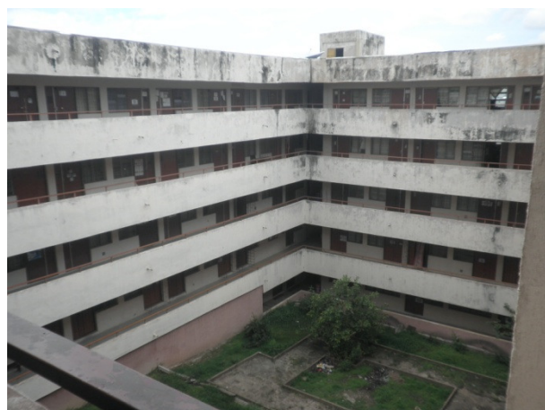
Plate 8: Defaced parapet walls (Author's survey 2012)
