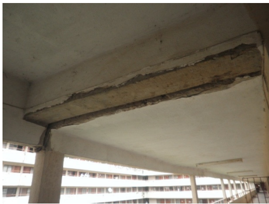
Plate 3: Damaged structural beam (Author's survey 2012)
