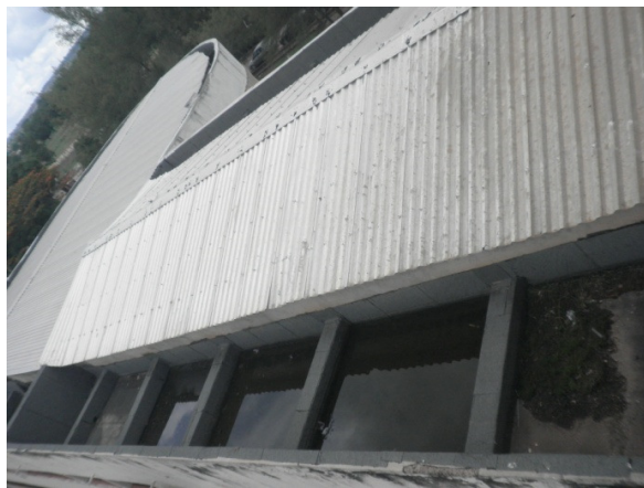
Plate 5: Accumulated water on the Roof gutter (Author's survey 2012)
