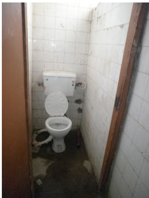
Plate 1: Poor state the of the toilet facility (Author’s survey 2012)
