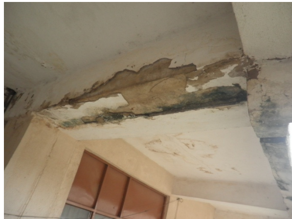
Plate 6: Defected expansion joint. (Author's survey 2012)
