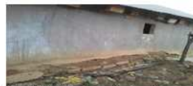
Plate IX: Chicken houses hung on the eaves of roof Source: Authors' Field Work 2013
