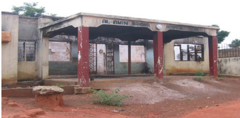
Plate 9: A Hospital Razed and Destroyed in Jos North, (Field Survey, 2011)
