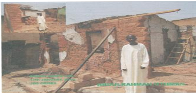
Plate 10: A House Burnt in Jos North, (Field Survey, 2011)
