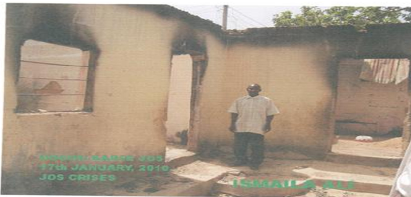
Plate 4: A House Burnt in Jos South, (Field Survey, 2011)
