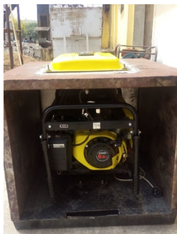
Figure 3: Enclosure and 2KVA Electric Power Generator
